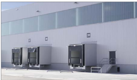
Installed on wall.
